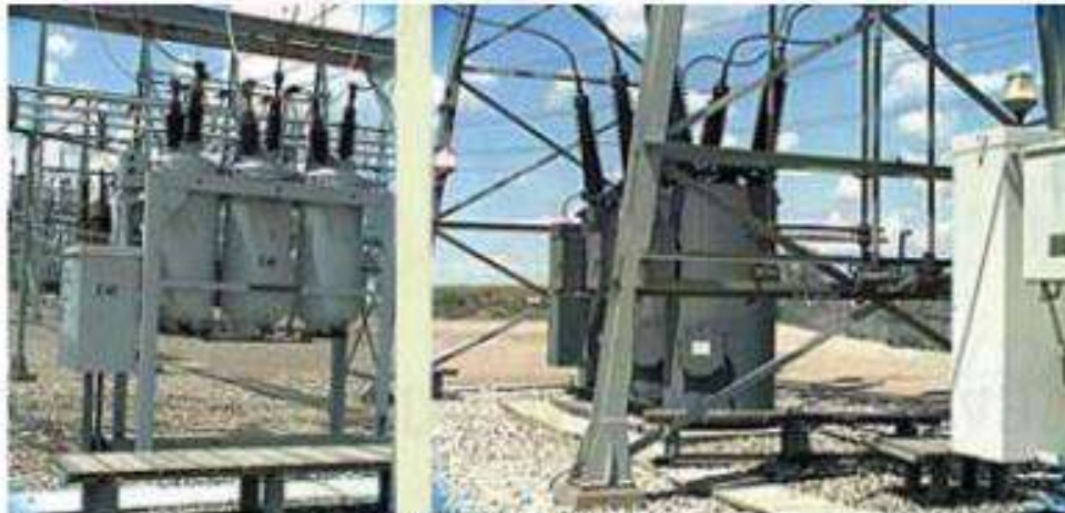
Oil Circuit Breakers
